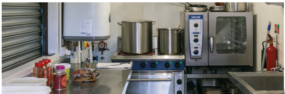
COMMERCIAL KITCHEN - Design & Build
