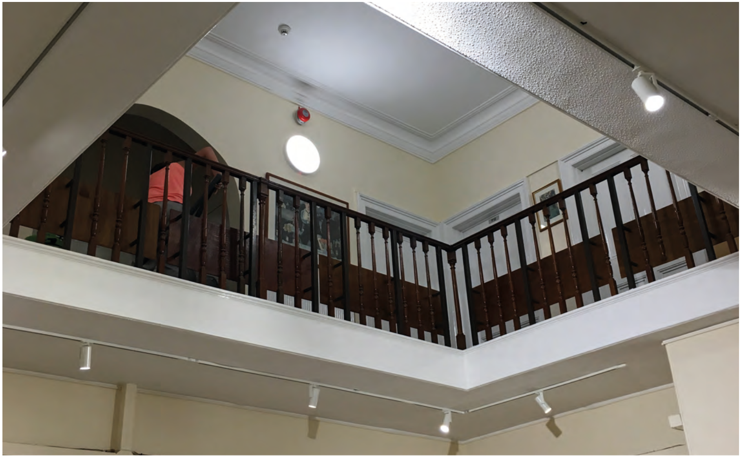
ATRIUM AREA - Track Lighting With Spot & Fixed LED Lights
