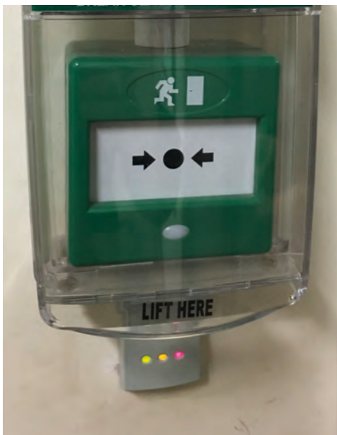
ACCESS CONTROL Main Entrance Door
